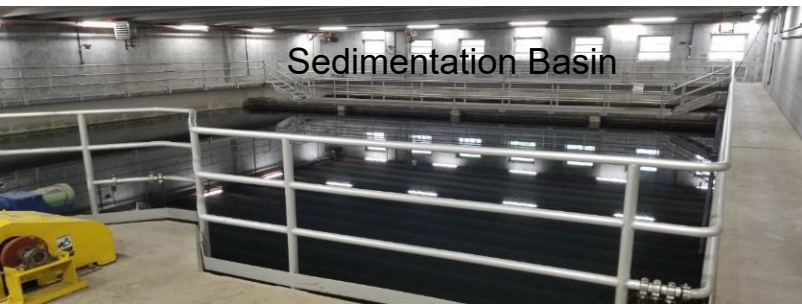
Flocculation Mixing Basins
