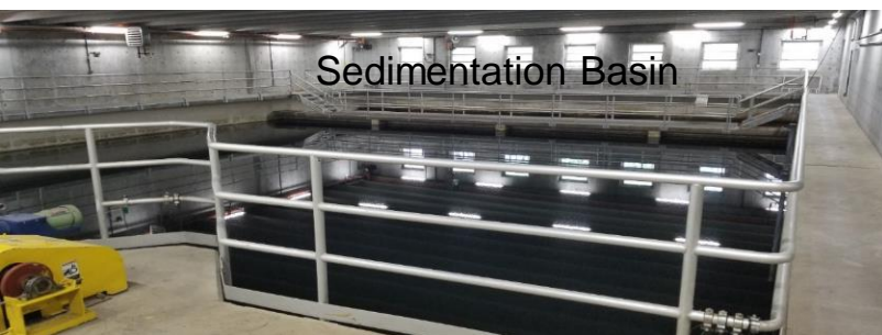
Flocculation Mixing Basins
