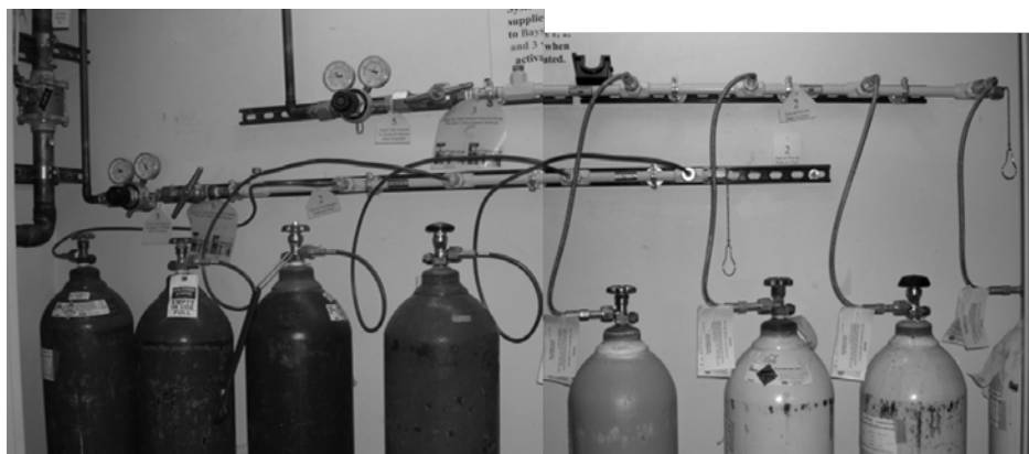
Figure 2: Existing reserve cylinder room at UIHC
