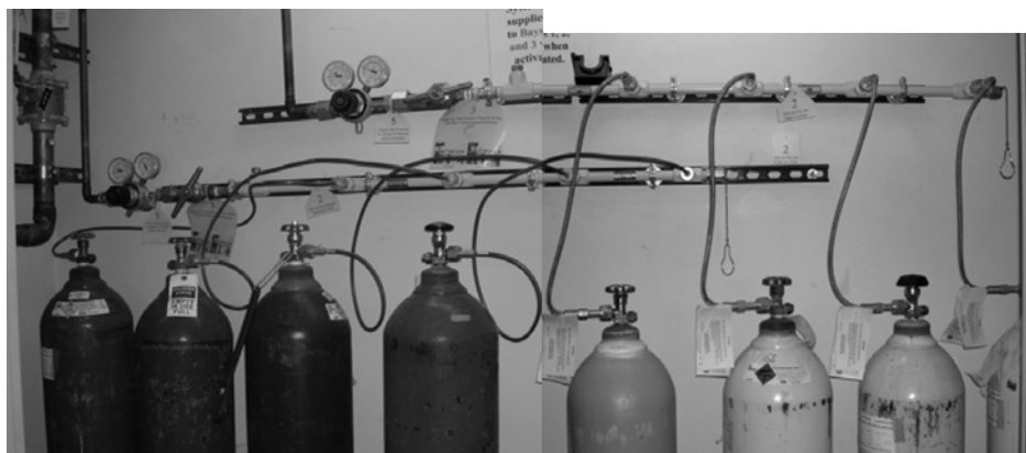
Figure 2: Existing reserve cylinder room at UIHC
