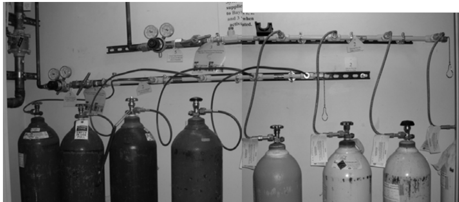
Figure 2: Existing reserve cylinder room at UIHC
