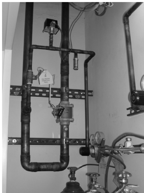
Figure 3: Existing reserve cylinder room at UIHC
